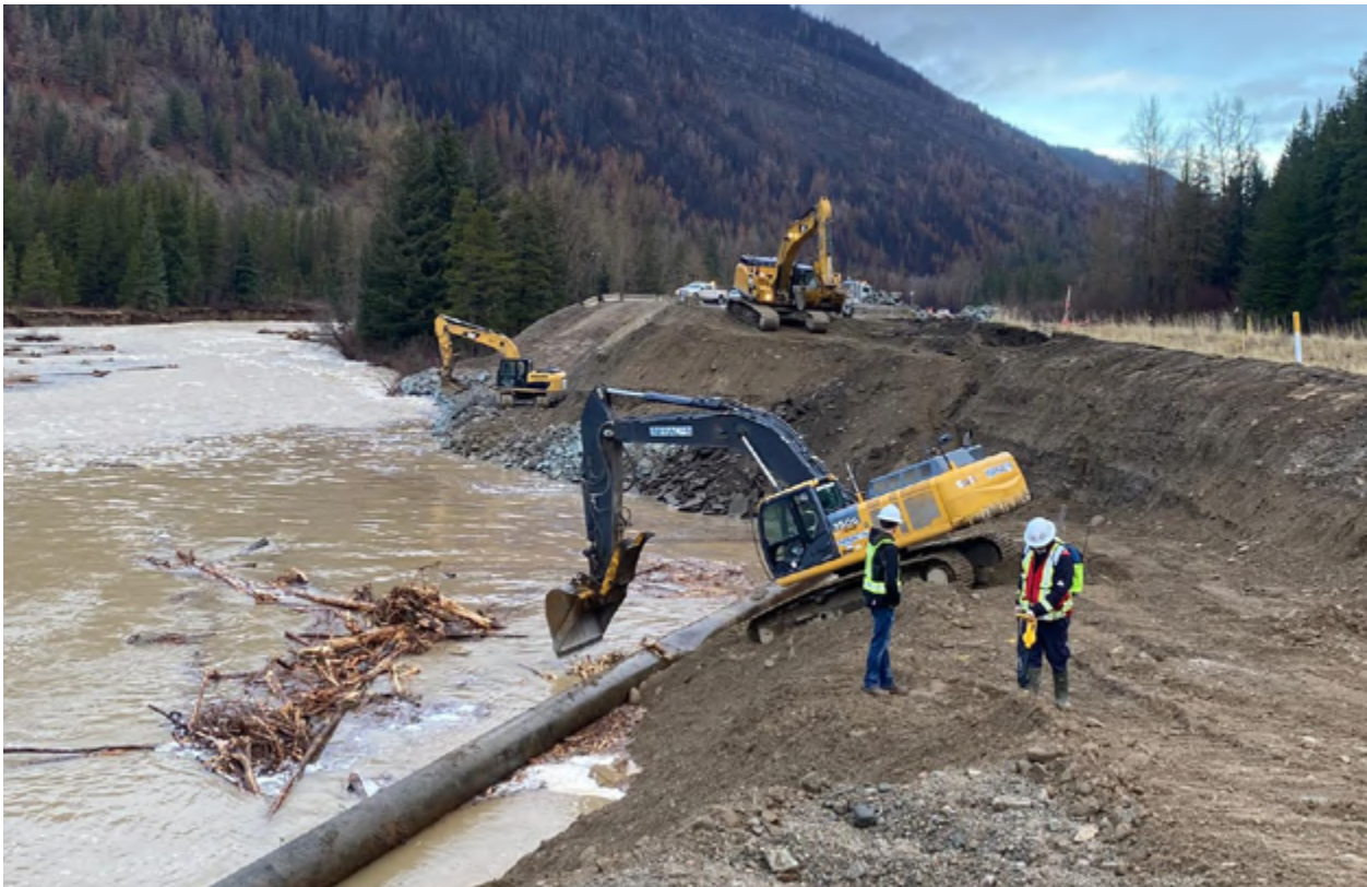
The Fraser Valley flood of 2021 exposed portions of the existing Trans Mountain Pipeline to the elements.
